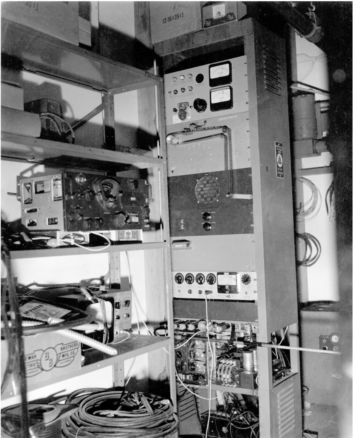
This is it, the original "WA6TDD Mt. Wilson Repeater" as installed in the back corner of the KPFK transmitter building on Mt. Wilson in 1962.
