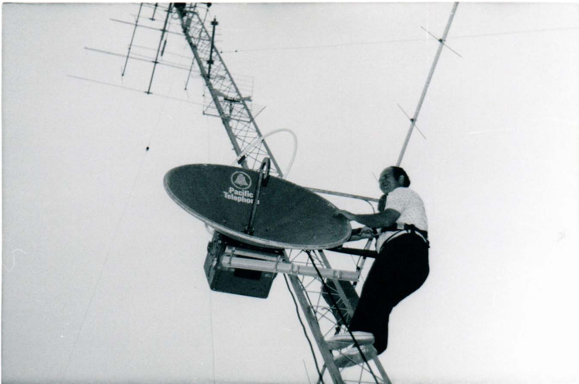
This is K6OQK on the tower at home making initial adjustments to the 4' STL transmit dish. The dish was just high enough to comfortably clear trees about two blocks away. The path length to Mt. Wilson was 26 miles.
