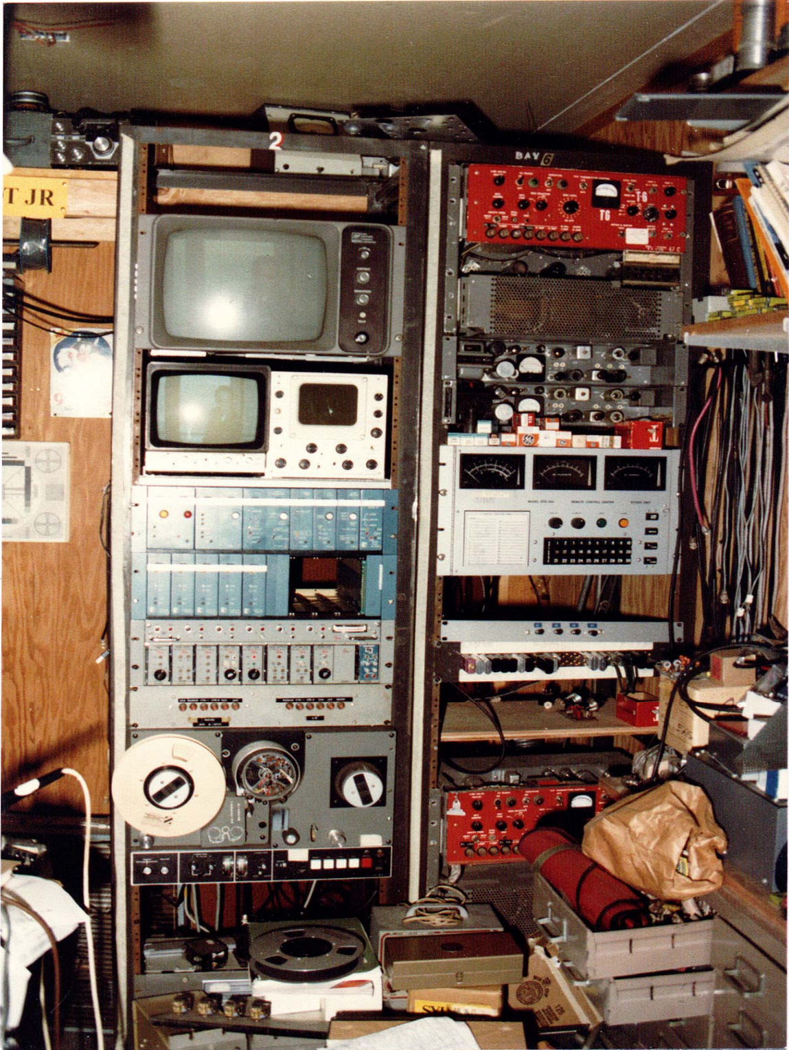
The WR6ABE / WA6TDD STL (Shack Transmitter Link) in Woodland Hills circa 1981. In the right rack at the top is the RCA TVM-1 Microwave transmitter control unit. Below that are the 6.8 and 6.2 MHz sound channels modulators, and below that is the Moseley PBR-30 remote control. The control unit in the bottom of the rack was a spare unit. The equipment in the left rack was video equipment that fed the microwave's video channel in the hopes that someday we'd figure out something fun to do with it.
